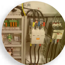
Elevator Control System Modernization
